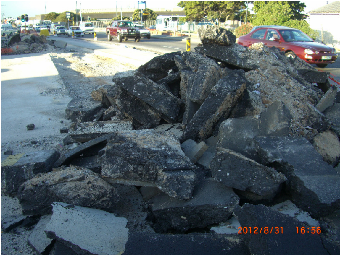
4. High quality of material removed, asphalt generally 150mm thick removed during demolition. This road surface was adequate for any kind of future traffic and should not have been removed. Painted lanes could have done the job on this high grade surface. This is part of the wasteful expenditure generally seen in IPTS works. Plans are created by consultants, who benefit from a fee structure, and are approved by Municipal officials who are non Transportation Engineers. Cost penalties are two fold, planning is outsourced to consultants at huge fees because Municipality does not have capacity, and Municipality is unqualified or unmotivated to guard against sloppy research and over specification.
